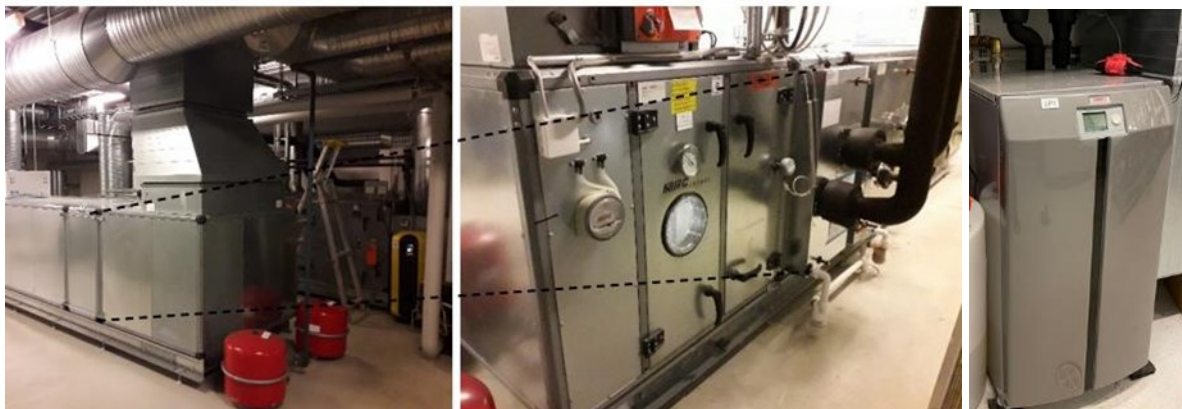
Figure 5: Exhaust air unit of washrooms and dressing rooms from different sides, additional heat exchanger installed (dashed lines indicate location); heat pump Gebwell T2 (right)
