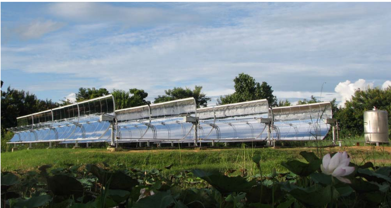
Fig 2 Solar Parabolic Trough Power Plant for 10 kWe (100 kWt)
